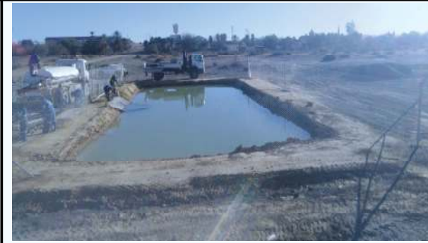
Photo No. 4: Fencing off tempory pond to meet Safety and environmental standards
